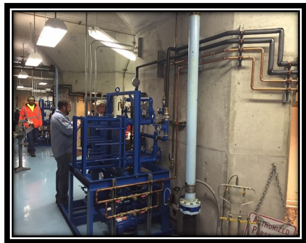
TGB Heat Exchanger & Pumps
