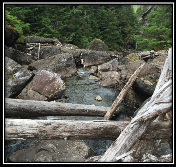
Weir Downstream Leakage 2015
