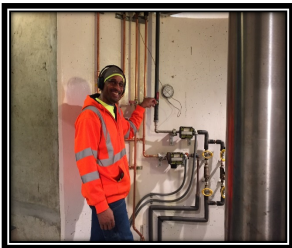
TGB Cooling System Valves
