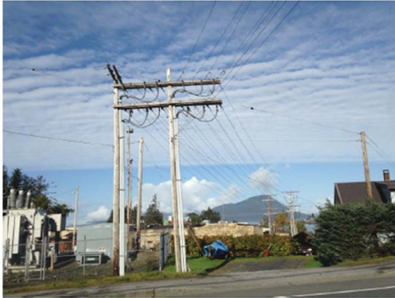
Wrangell Distribution "H" Structure (central tie-in point for all electrical services in Wrangell)
