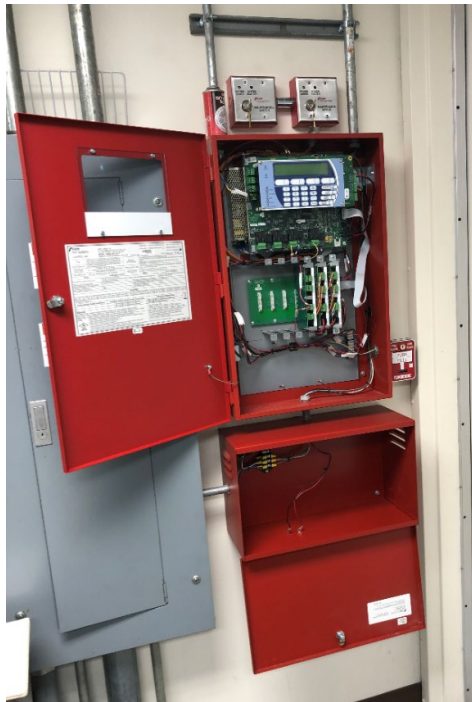
Kidde Aries Series Fire Control Panel During Installation
