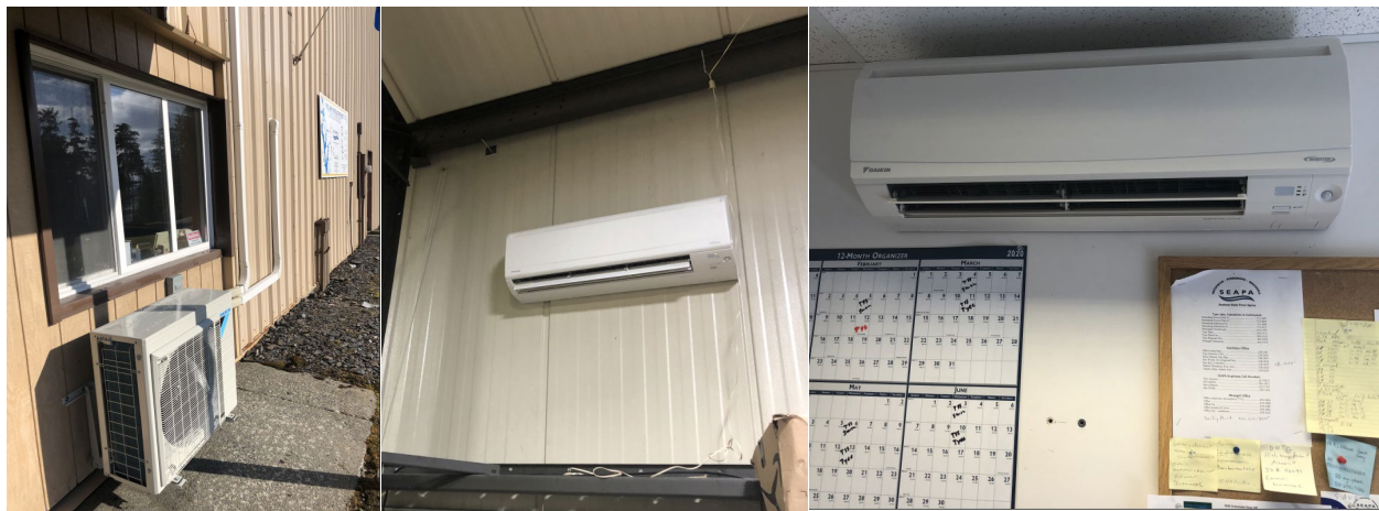
Daikin Heat Pump Wrangell Warehouse
